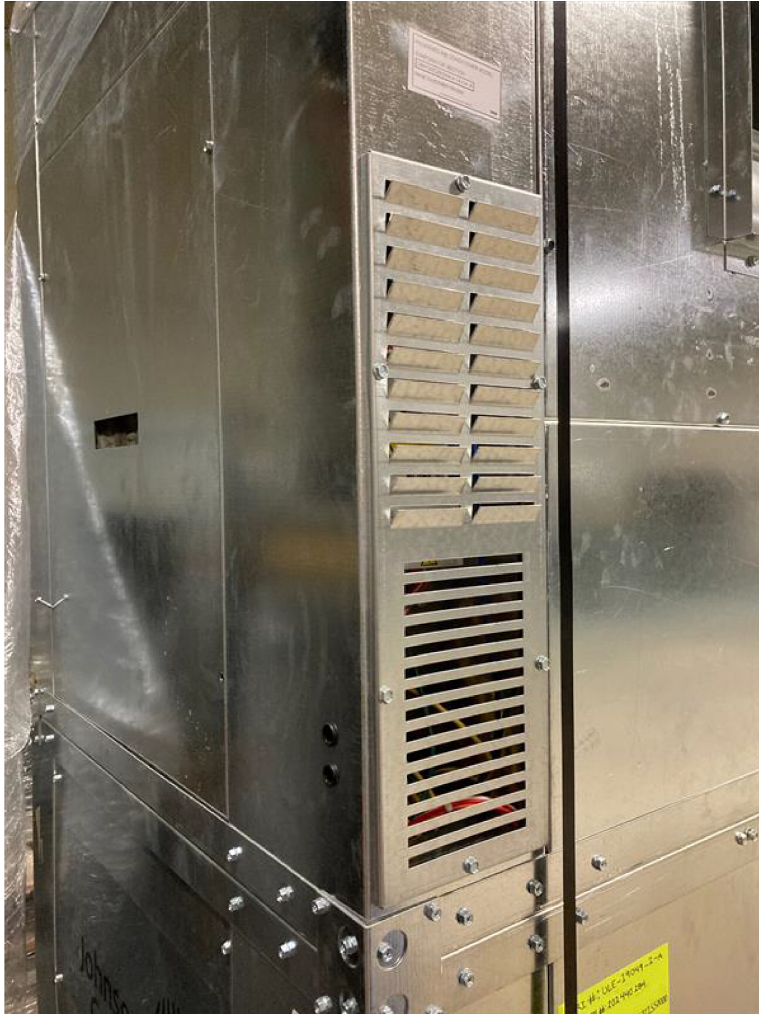
Figure 7: VFD grille cover
