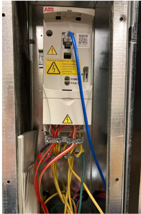
Figure 5: Internally routed ethernet cable
